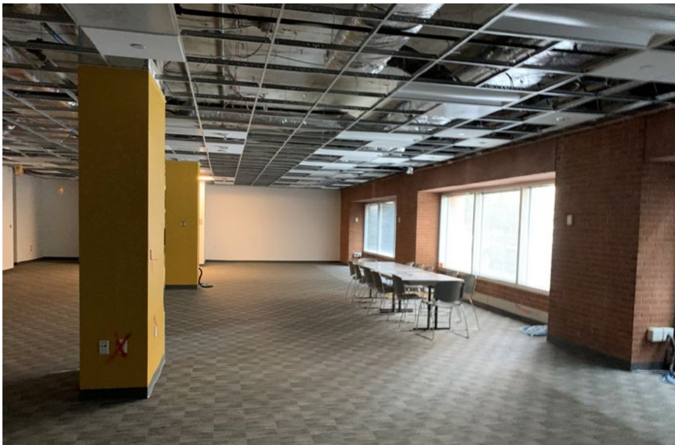
Reduced occupancy of office buildings can result in stagnant water in building plumbing systems.
